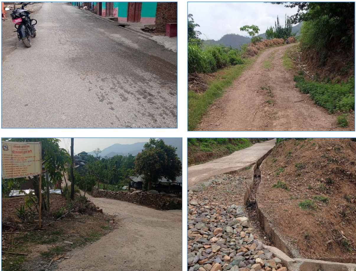
Figure No 4.6: Rural Road Condition
